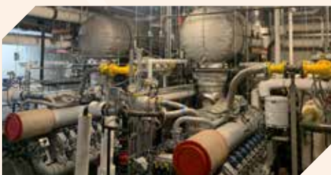
The cogeneration plant is powered by two natural-gas-fueled 1.5 megawatt units.
